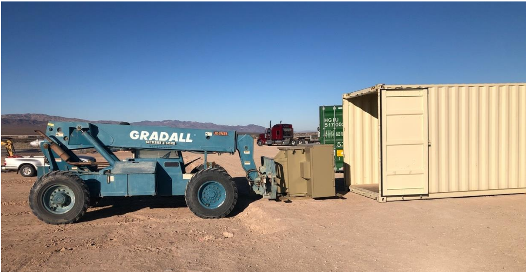
Figure 2: Delivery of Power Distribution Transformer
